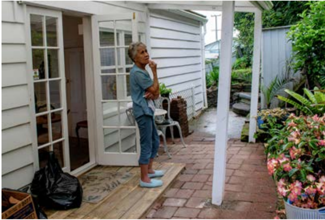
Nelly with the displaced cobblestones in the back garden. TOP RIGHT: The damaged corner where the floorboards heaved, and the Tararu home.
