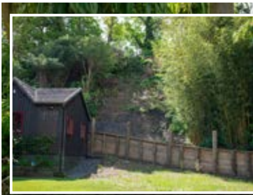
Donna Pervan is concerned discharge from a stormwater drain could cause damage to iconic Thames walkway Jacob's Ladder, or slips on to the property where she lives. ABOVE: The new retaining wall behind the garage.
