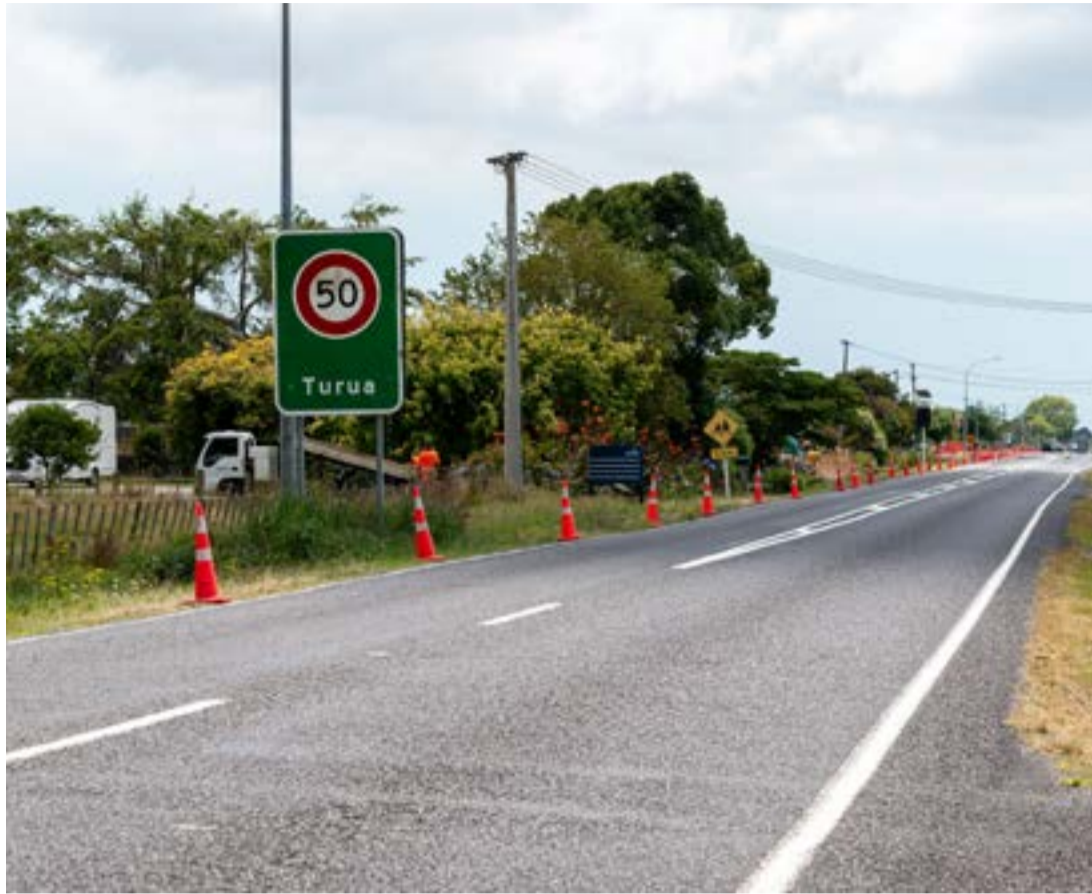
Pavement rehabilitation works on Hauraki Rd are being undertaken at the same time as the Onetai Stream Bridge replacement on SH26.
