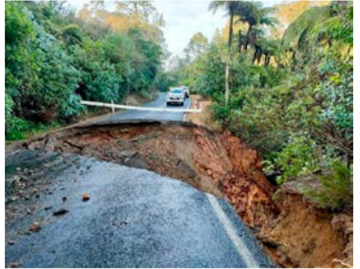
Golden Valley Rd was damaged in May, 2023. Photo: SUPPLIED/HDC
