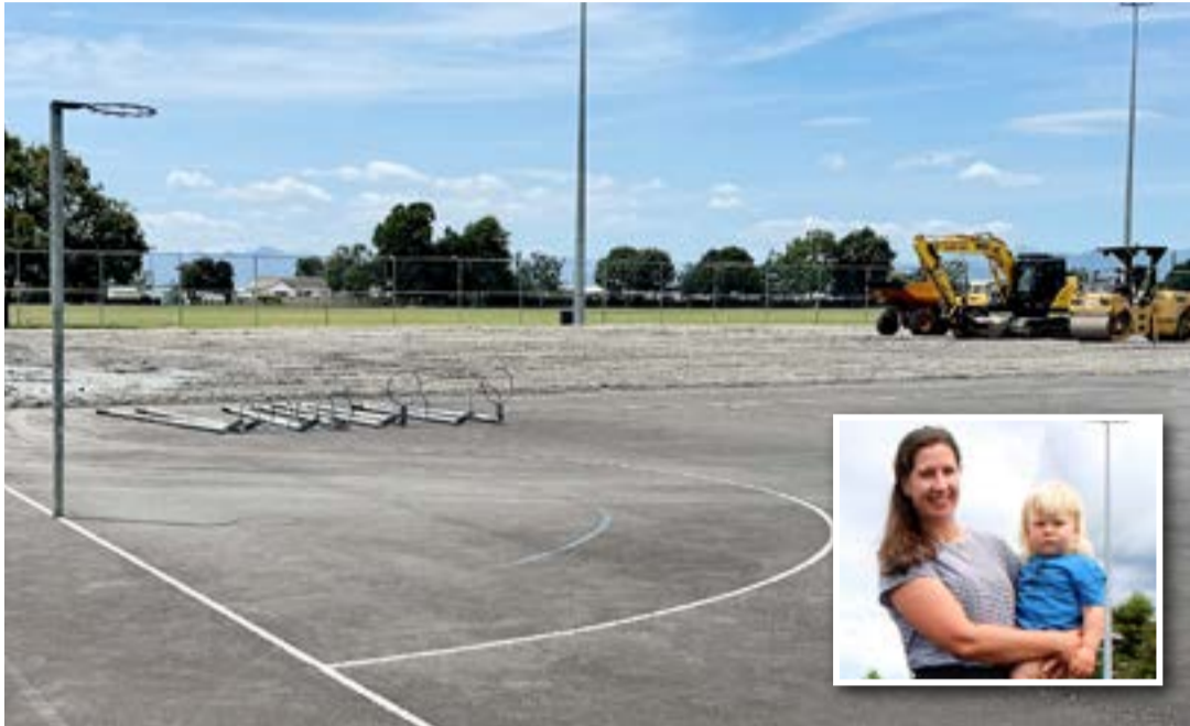
Work to resurface four of Ngātea's netball courts is underway. INSET: Fundraising officer Tara Carter. Photo: SUPPLIED
