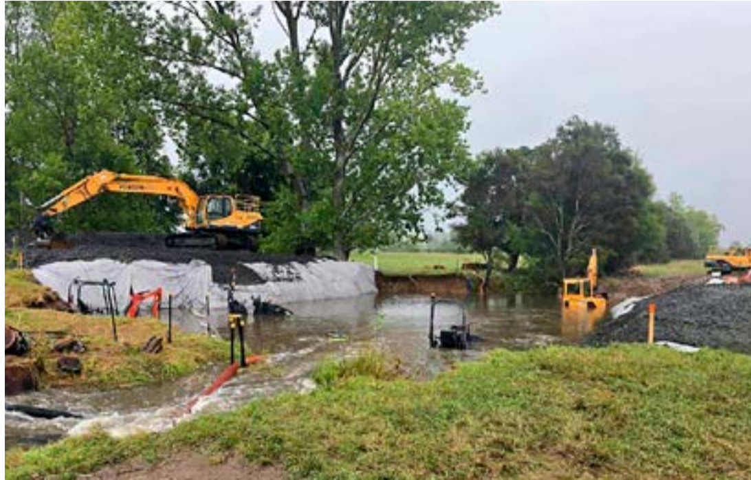
Equipment was flooded at the worksite after being left along the streambed during a storm. RIGHT: A temporary pedestrian bridge has been constructed through the worksite for local school kids.
